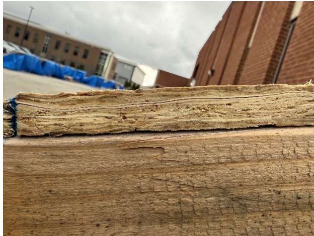
Figure 9. Swelling of OSB panel edge following the first rain event.
