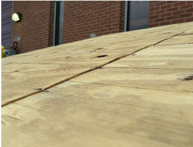
Figure 8. Swelling of plywood along the edges of the panels following the first rain event.
